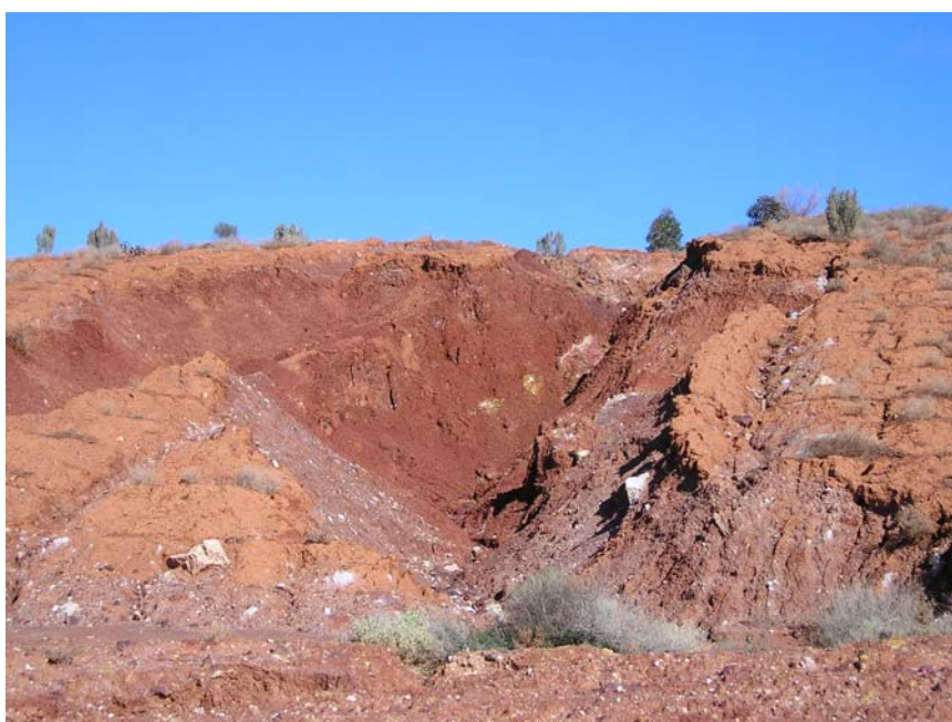
Figure 2. Tunnels collapse forming a large gully.
